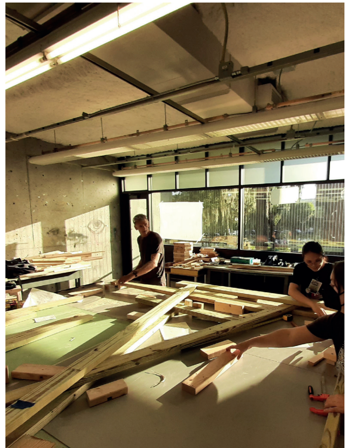
Figure 6 Laying out a finalized bent in the jig at School of Architecture.
